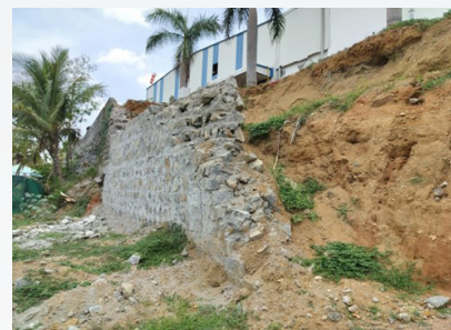
Image of the UCR Wall that has collapsed due to rain.
