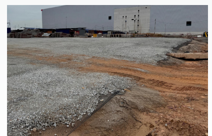
Road base construction underway at Daiso warehouse distribution centres with Multiaxial geogrid
