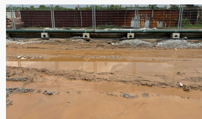
Waterlogged soil with poor drainage and exposed pipes. Thick soft clay subgrade issue before construction
