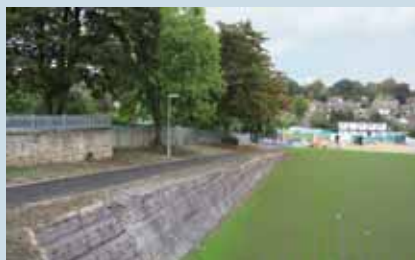
With construction successfully completed, the Tensar tech GreenSlope can be prepared for the vegetation stage.
